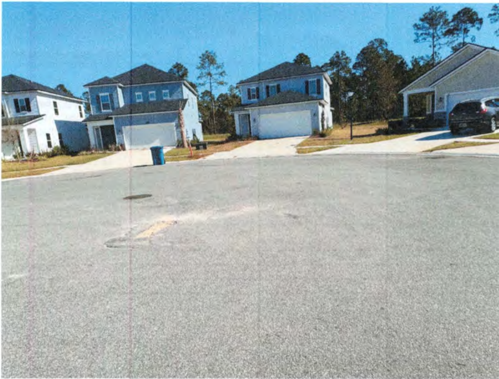
Pothole in the cul-de-sac of Bermudez Way.
