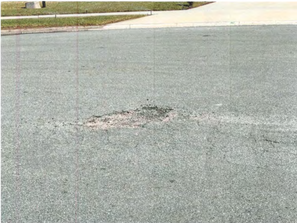
Pothole in the cul-de-sac of Torres Trace.
