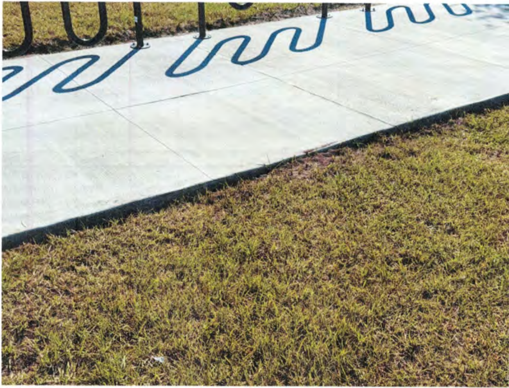
4" Drop off condition around bicycle rack sidewalk of 4" at the corner of Cordova Palms and Bermudez Way.
