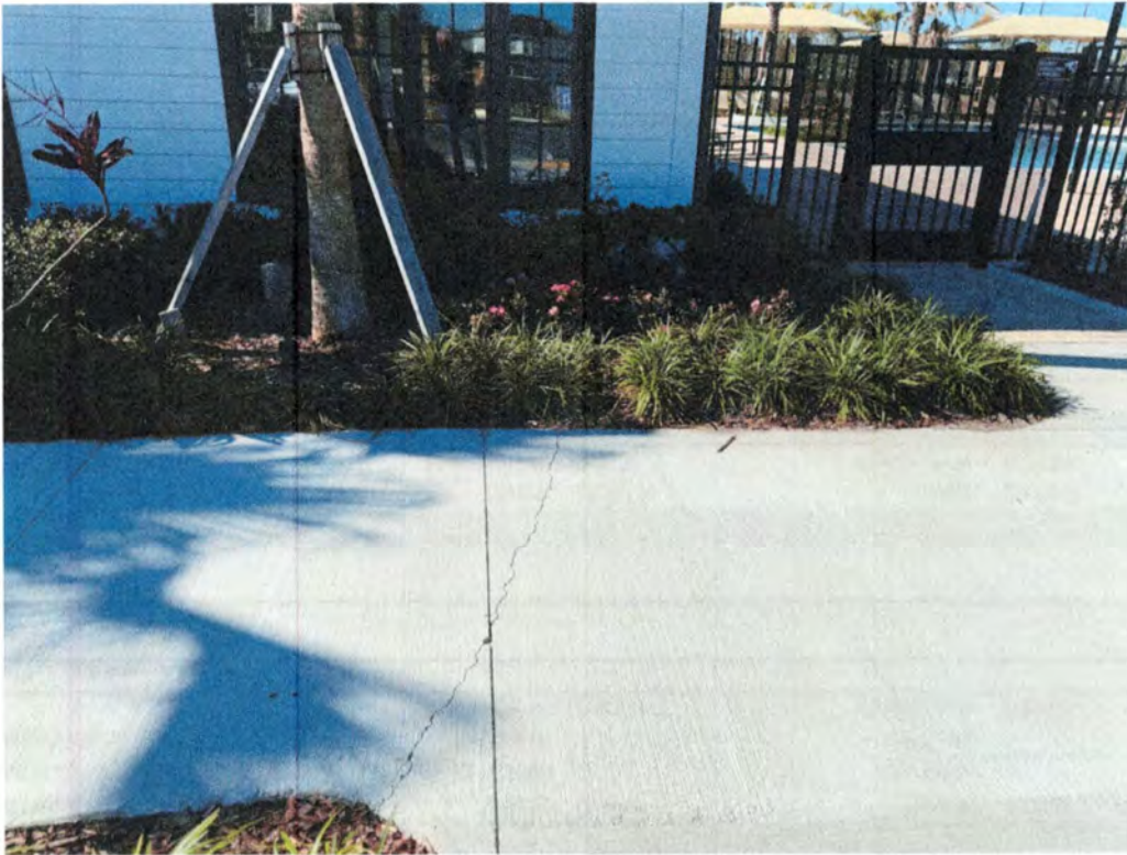
The sidewalk on the right side of the amenity center cracked.
