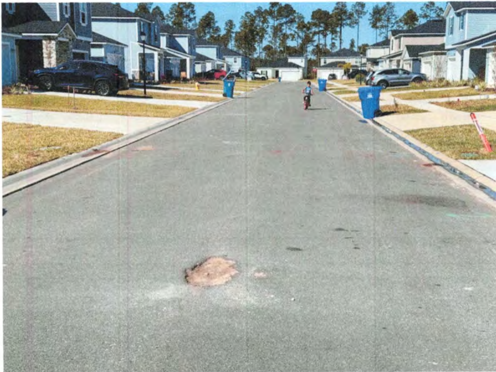
Pothole in asphalt at Posados Lane and Bourmount road.
