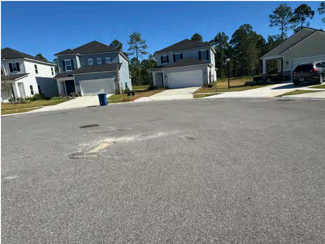
Pothole in the cul-de-sac of Bermudez Way.
