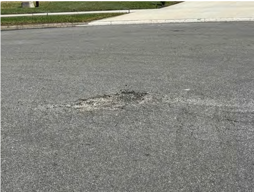
Pothole in the cul-de-sac of Torres Trace.
