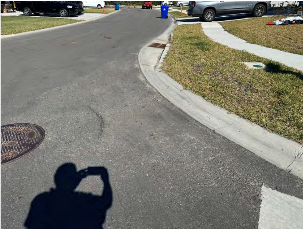
Asphalt failing possible storm drain failure, intersection of Barbosa Trail and Beaumont Road.
