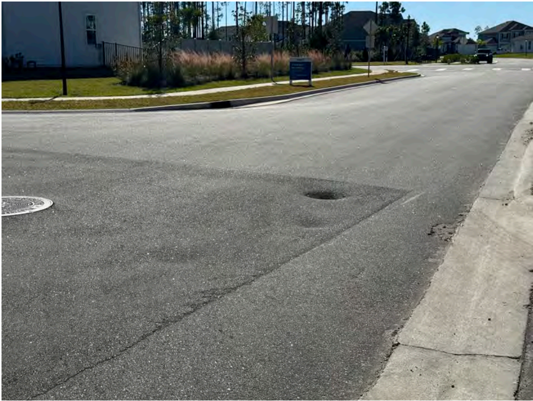
Pothole in front of the amenity center in an existing patch.
