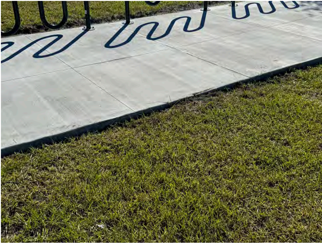
4" Drop off condition around bicycle rack sidewalk of 4" at the corner of Cordova Palms and Bermudez Way.
