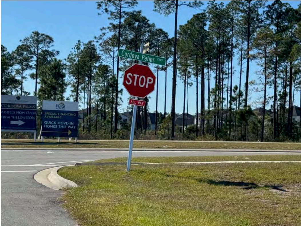
Stop Sign leaning at the Cordova Palms Parkway and S.R. 313.
